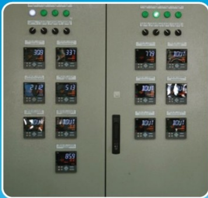
Heat Control Panel For Chemical Reactors
