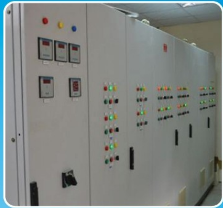
SCADA Controlled MCC Panel for Chemical Plant
